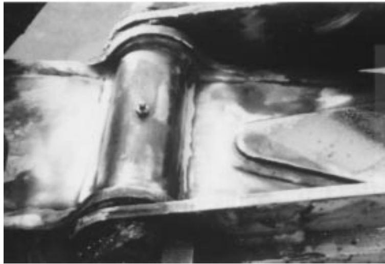
FIGURE 24.1: Fatigue cracking at welded detail in crane boom.
