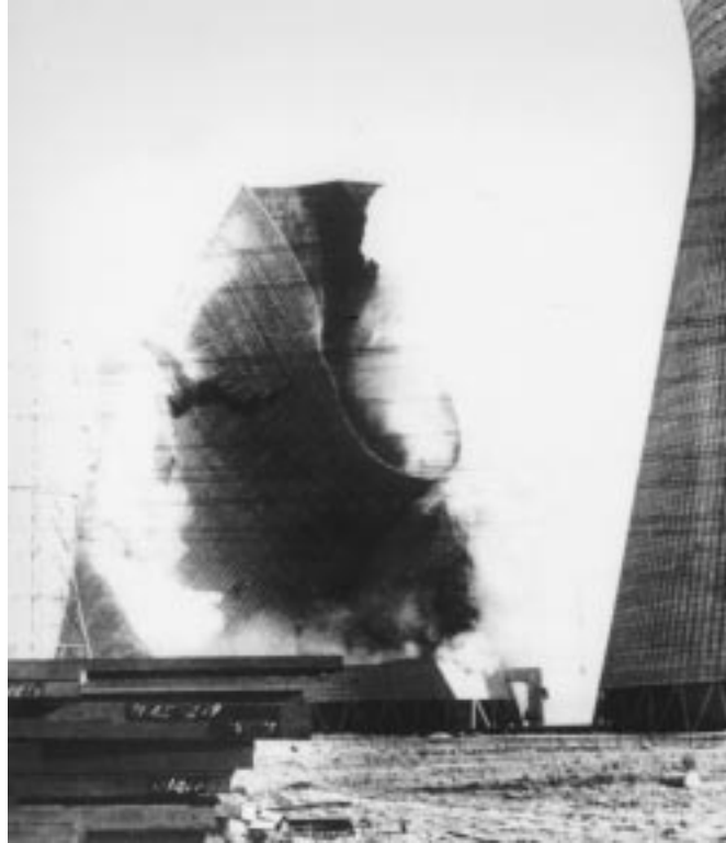
FIGURE 14.8: Collapse of Ferrybridge Power Station shell.
