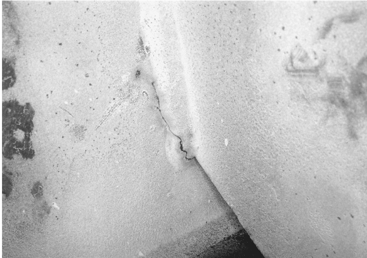
FIGURE 53.6 View of crack in the fillet weld joining the diaphragm connection plate to the web of a box section in the Washington Metro elevated structures. The crack is caused by distortion in the small gap between the bottom of the attachment plate and the box girder flange.
