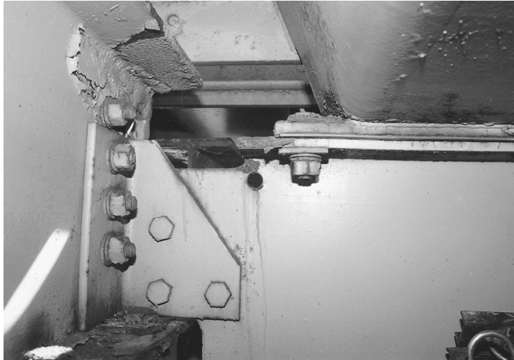
FIGURE 53.5 View of floor beam of Throgg's Neck Bridge in New York showing crack in the cope that has been repaired by drilling a stop hole. The crack is caused by incompatibility between the curvature of the superstructure and the orthotropic steel deck that is bolted onto the floor beams.
