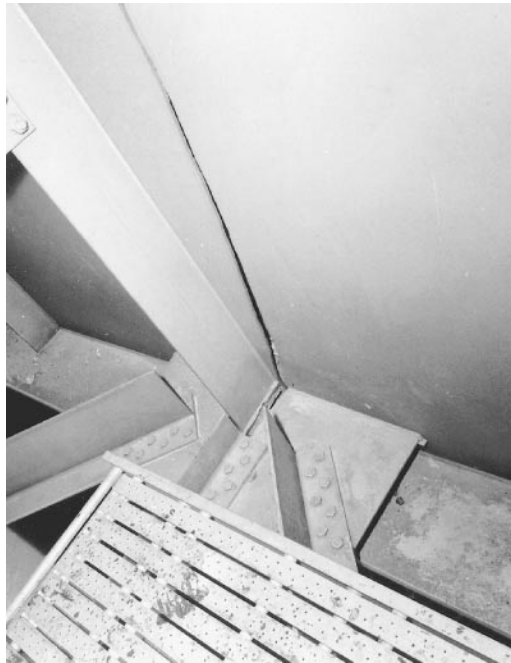
FIGURE 53.1 View of cracked girder of Lafayette Street Bridge in St. Paul, MN showing fatigue crack originating from backing bars and lack of fusion on the weld attaching the lateral bracing attachment plate to the web and to the transverse stiffener.
